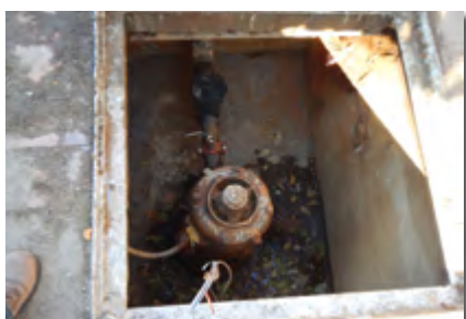
Production well vault - pre-abandonment.
