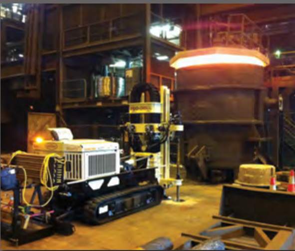
PRO-DRILL uses their 6622CPT rig in the Glenbrook Steel Mill pushing up against one of the melting pots in Glenbrook, Auckland in New Zealand. The temperatures were so hot inside that the computer screen on the rig went black, but, according to Kris Hines, PRO-DRILL Driller and CPT Operator, "the rig never skipped a beat."
