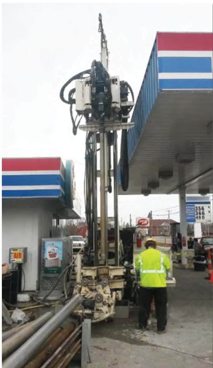
Bryan Marshall, Driller for Stearns Drilling, uses the 8140LS to install a monitoring well between a building and service station canopy. This mid-sized sonic rig from Geoprobe Systems® can easily maneuver into confined areas with minimal disturbance to the surroundings.
