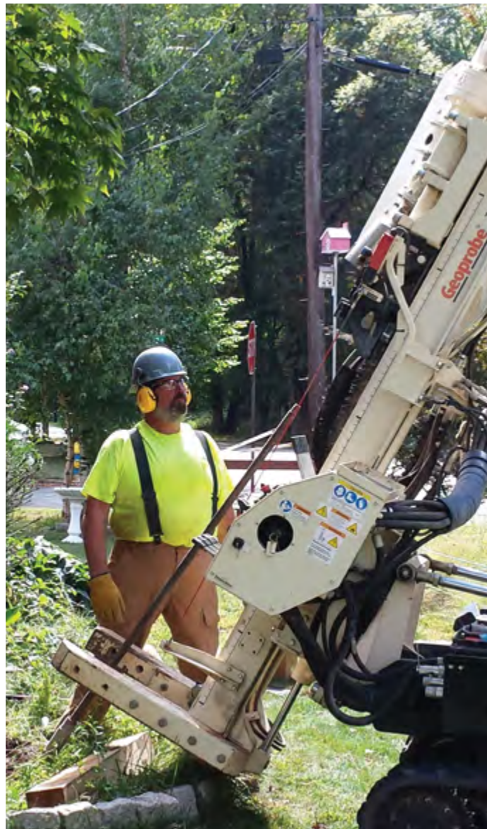
Doug Turner uses a 7822DT to inject Humics, an in-situ chemical beneath a building, through an angle boring. Drilling through the basement at this commercial building was not possible because the floor had radiant heat in the slab, the basement was an office with limited height, and most importantly, the business did not wish to be disturbed and denied basement access.
