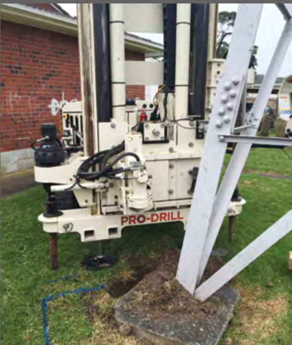
Pile bell testing on power pylons. Testing was done at 100 mm and 200 mm off the face of the pile. PRO-DRILL was able to complete the testing because of the 6622CPT rig's unique anchoring and pushing configuration at the front of the rig and not in the center like other CPT rigs. The investigation was done to show that any uplift against the pile bell had not weakened the ground above the bell, and to help in designing new foundation improvements to support heavier power transmission lines.
