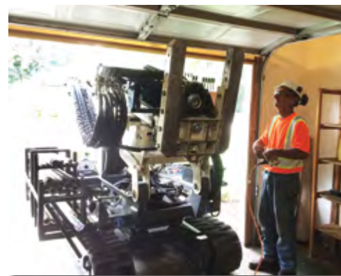
Rob Mores drives the 6712DT into a residential garage with a 7-ft. overhead door clearance.
