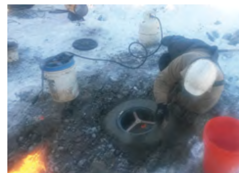
Bryan Marshall, Crew Chief/Driller for Stearns Drilling, works at installing a 2-in. monitoring well using cold weather 'techniques' while pouring the concrete.
