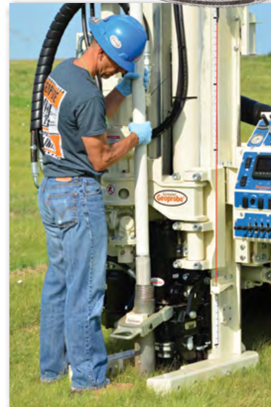
Lee Shaw, Geoprobe® Sales, uses a 7822DT to install a new 2.0 in. Slim Prepack using new 3.75 in. Tooling.
