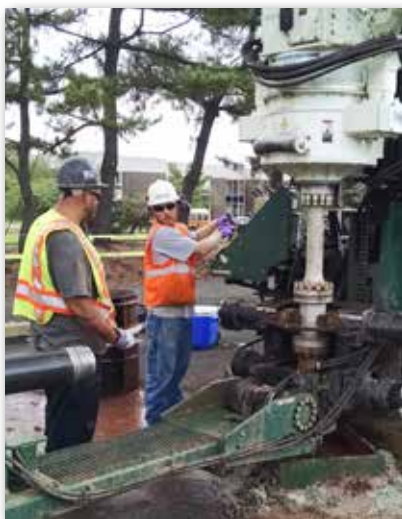
Jason Kuni (left), Lead Driller for Enviroprobe Services, and Jed Davis, Geoprobe® Tools Engineer, work at the 420-ft. boring site testing the new Geoprobe® SDT60 (Sonic Dual Tube 6-in. system).
