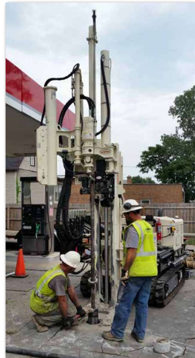
Daniel Fisher (left) and Robert Albinger, Horizon Construction & Exploration, remove the inner drill string to allow an open and cased hole for easy installation of Cathodic Anode.
