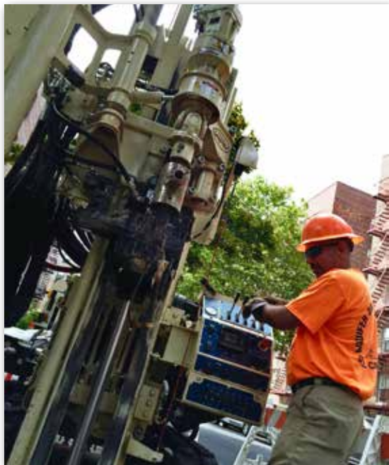
ADT added four new Geoprobe® 7822DTs to their fleet for the NYC Green Infrastructure Plan because of their compact size and easy maneuverability. Chris Migliore, ADT Driller, is at the controls of this rig.
