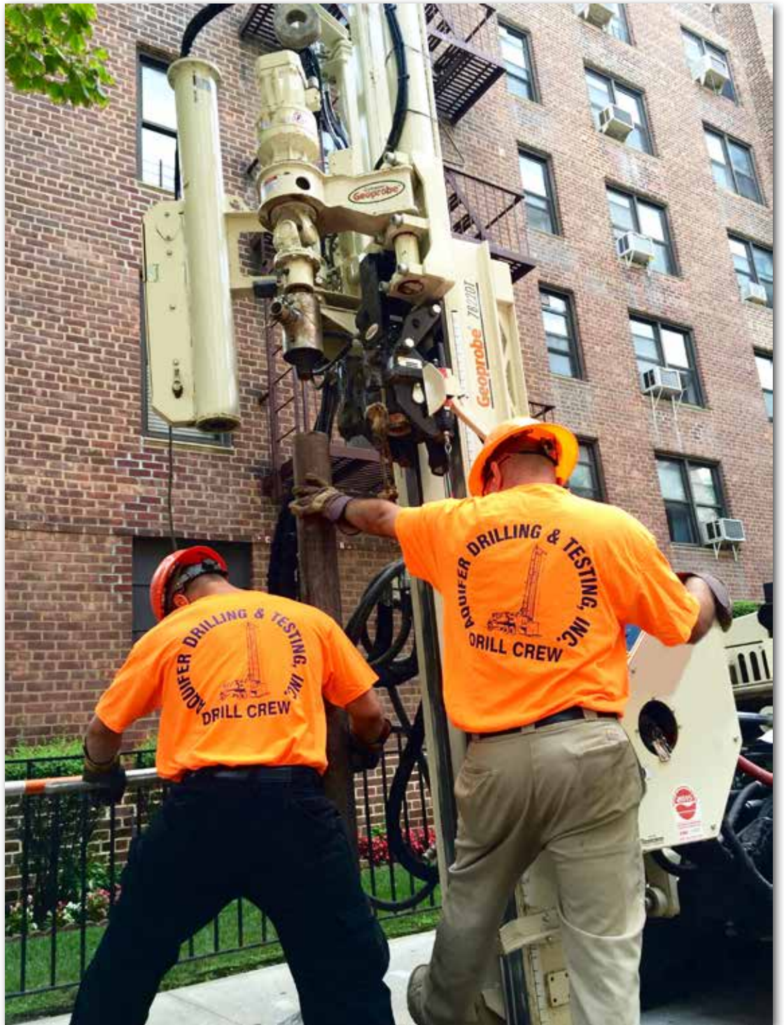
James Corsitto (left), Helper, and Chris Migliore, Driller, run the ADT 7822DT rig. ADT has outfitted their 7822DT with a Side Port Swivel so they can quickly switch from direct push to wet rotary.
