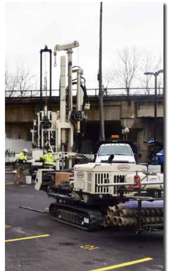
Horizon drillers utilized both of their Geoprobe® machines, the 3230DT and 7822DT on a project in Wisconsin.
