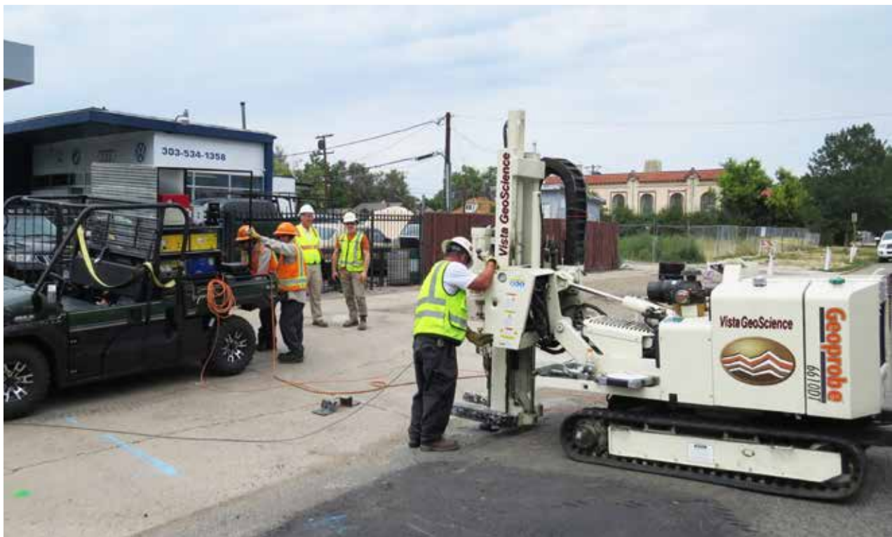
A Vista GeoScience field crew runs MIP (Membrane Interface Probe) and OIP (Optical Image Profiler) systems at a former gas station site in Denver, CO. Vista mounted their new MiHPT and OIP systems in a self-contained, steel pallet rack system which slides into the back of a 4WD ATV allowing maximum mobility and access on more difficult sites.
