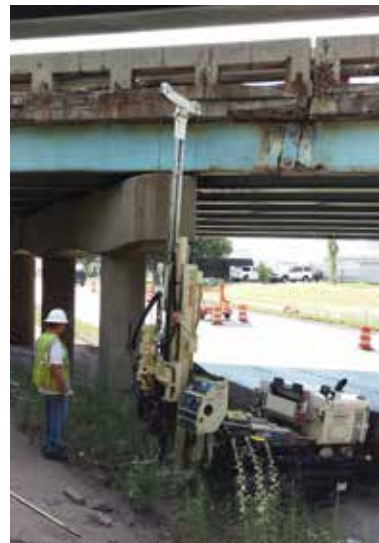
John Deitrick, Driller, and the Stearns Drilling 7822DT retrieve soil samples for a future I-75 bridge reconstruction project in Allen Park, MI.
