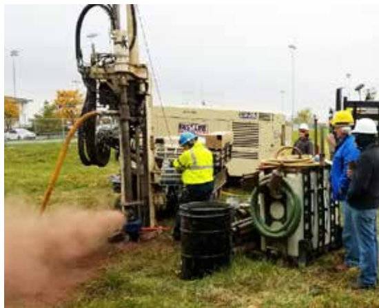
Dave Latimer, Driller with EPI, runs 6-in. air with a 7822DT to 85 feet based on water levels determined during the project.
