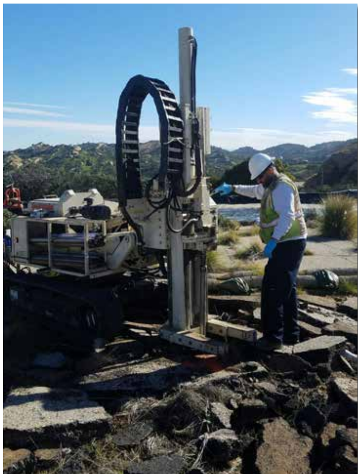
Eric Herrera, Driller for Strongarm Environmental, uses the 6620DT to tag bedrock.
