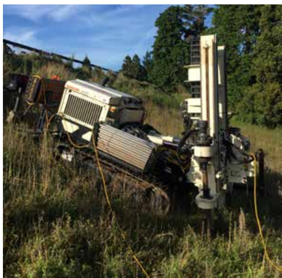
Having the ability to set up the mast vertical while the tracks follow the slope of the terrain has given Pro-Drill the ability to perform soundings on hill faces and on dam faces without the need to dig in tracks or platforms.
