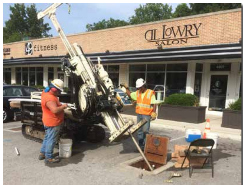
Toby Mielenz (left) and Rob Mores use a 7822DT for angle probing to install 1-in. sparge wells.
