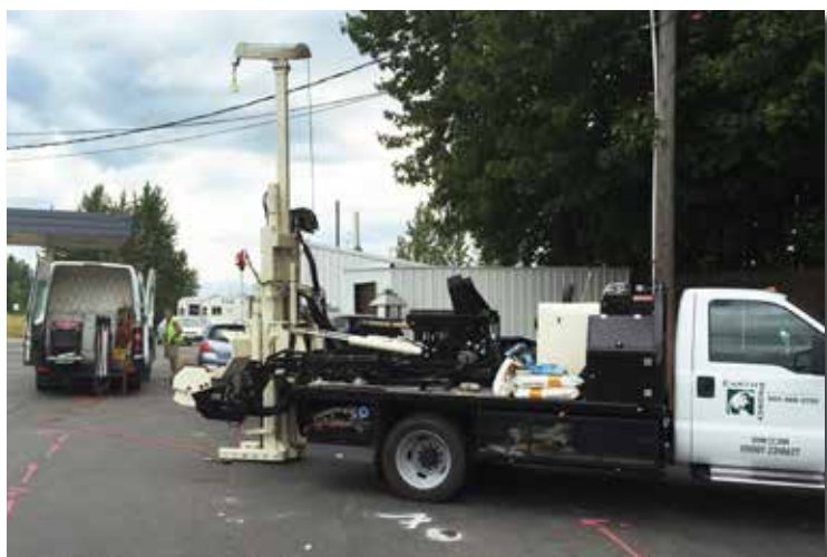
Sandpoint, ID. Supporting UVOST/MIP/HPT direct sensing investigation and confirmation soil sampling with a Geoprobe® 7800.
