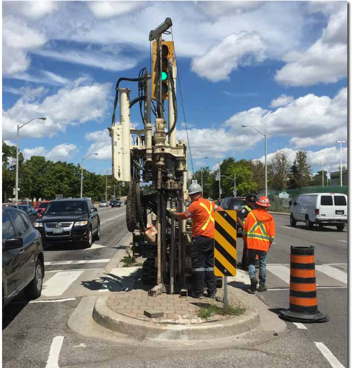
The small footprint of the 7822DT allowed Landshark Drilling to operate at a busy intersection in downtown Toronto. The 7822DT averaged 270 feet per day of direct push for the large infrastructure project.
