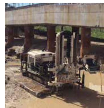
Working on swamp mats for post testing of ground strength after driven wooden piles were used to improve ground conditions for a bridge construction on state highway upgrades.
