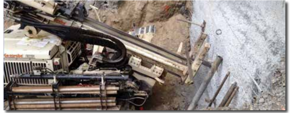
One of Landshark's 7822DTs is angle drilling a directional boring for tiebacks.
