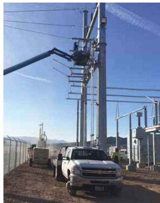
Subsurface work was completed at the same time a new substation was constructed at each of the three sites.
