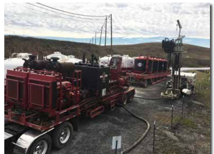
An oilfield cement pumping unit was used to pump cement slurry during the abandonment process. In all, nearly 20,000 gallons of slurry was used. The 8150LS (right) was used to penetrate the concrete pipe in the lagoon.
