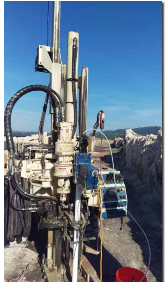
With 30-ft. ash ponds on either side, a 7822DT, with a tubing pump (and check ball), collect SP16 groundwater samples from between 50- to 60-ft bgs. The machine is located on a road between ash ponds with 3-foot-high berms.
