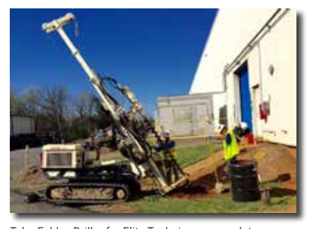
Tyler Felder, Driller for Elite Techniques, completes an angled well installation in upstate South Carolina.
