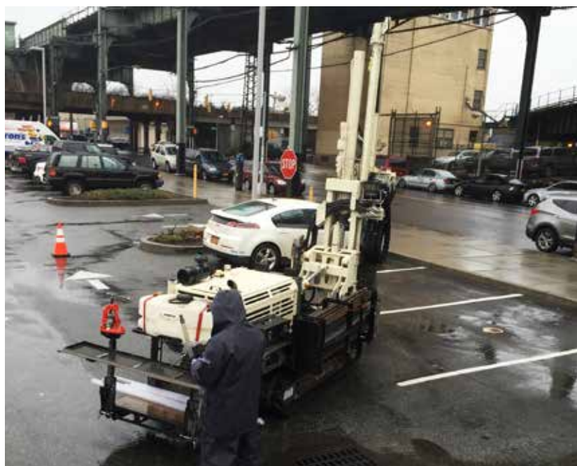
Retail businesses in the area were able to continue with operations without interruption throughout the remediation installation process. Steve Bitetto preps the 6712DT for the next installation location.
