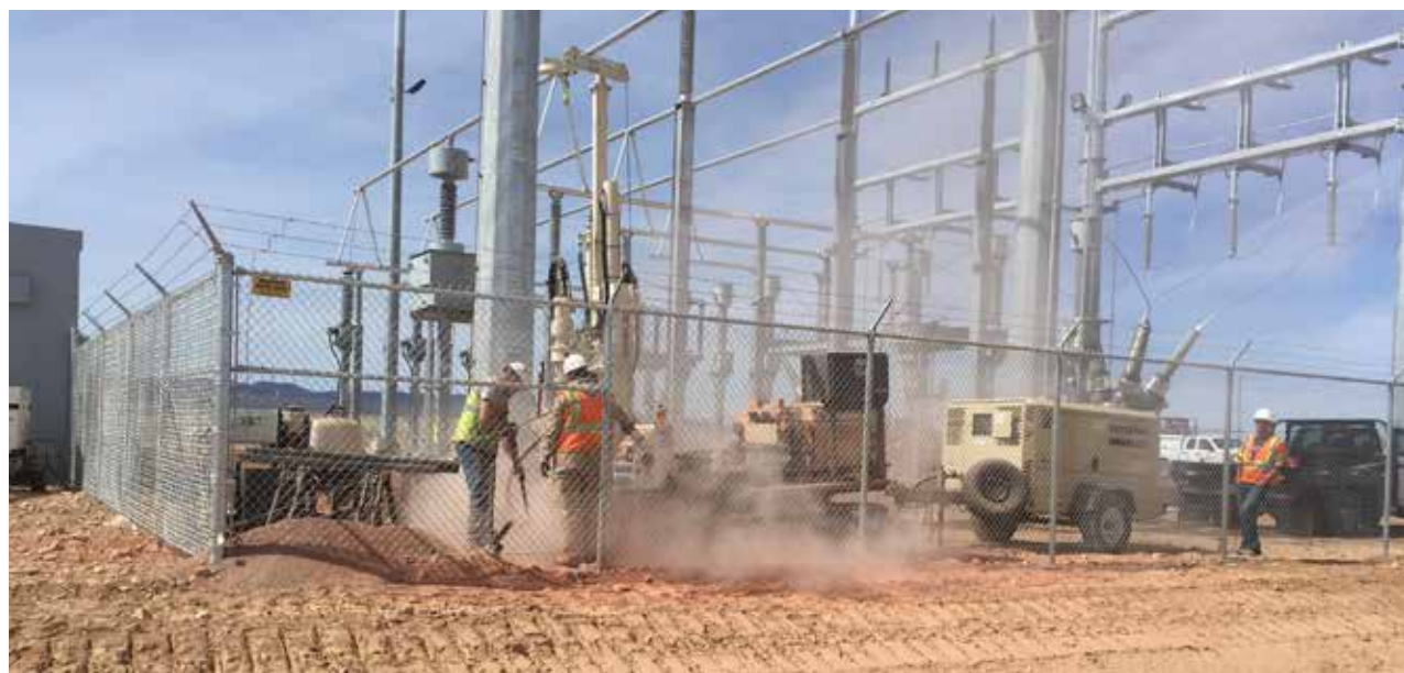
The new grounding rods Direct Push Services installed for the Utah solar grid project will help meet the demand for more power in the state.
