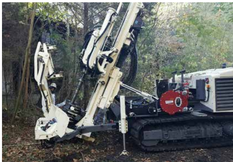
Angle drilling and the rod handling system show the capabilities of the 8150LS sonic.
