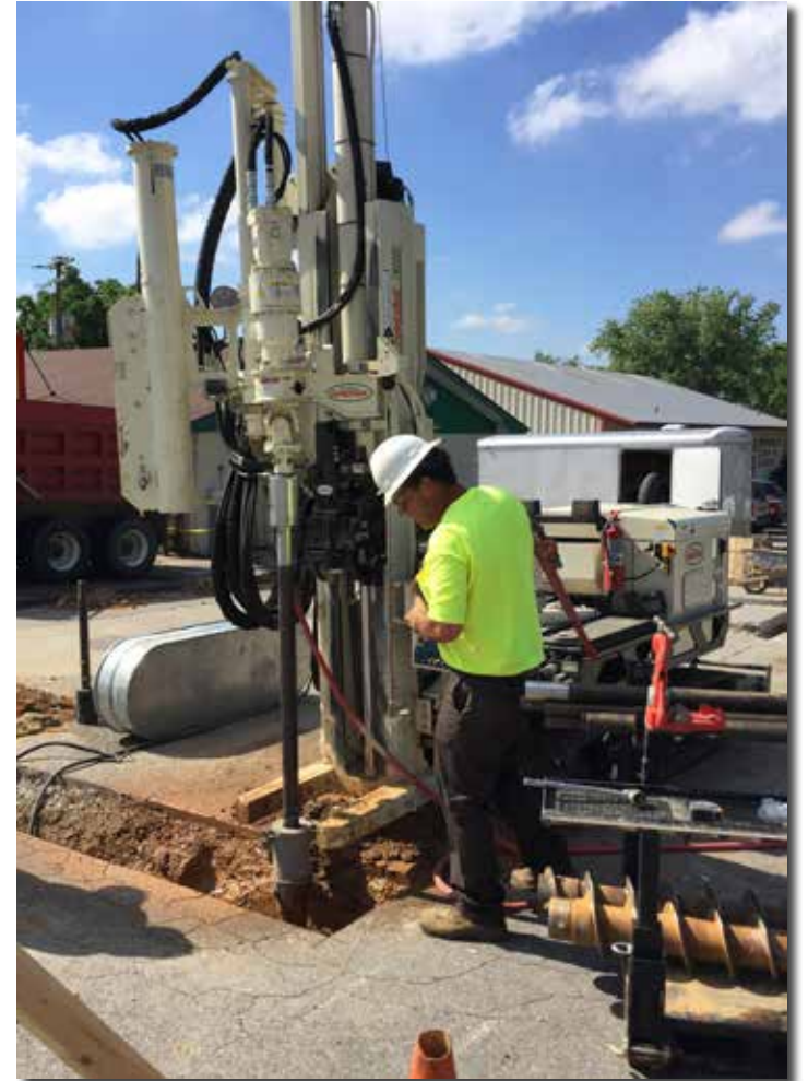
CORTEK Drilling in Spring Hill, TN, installs monitoring wells at a UST using air rotary.
