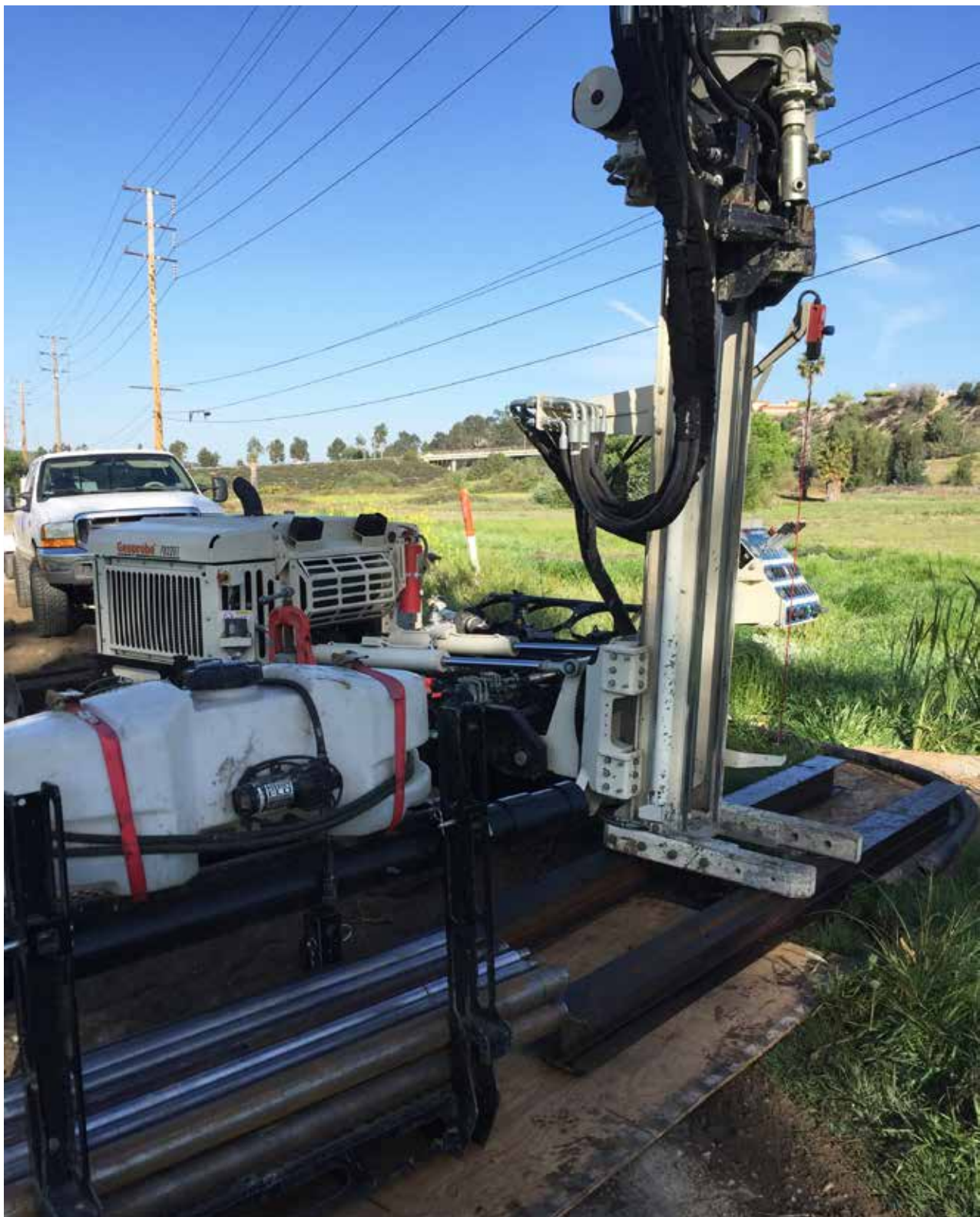
With 'I' beams and plywood sheeting for stabilization, the 7822DT is ready to plug one of several leaky abandoned CPT boreholes. One of the abandoned boreholes had grown up to 9-in. in diameter at the surface, and had a flow rate of about 6 gpm.
