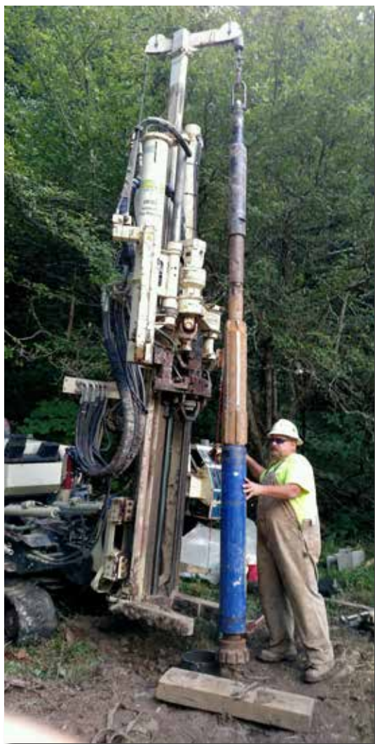
Chris Chronister, Field Superintendent for Eichelbergers, uses a 7822DT and a tool string with 8-in. air hammer and stabilizer to install a water well in a remote, protected area.
