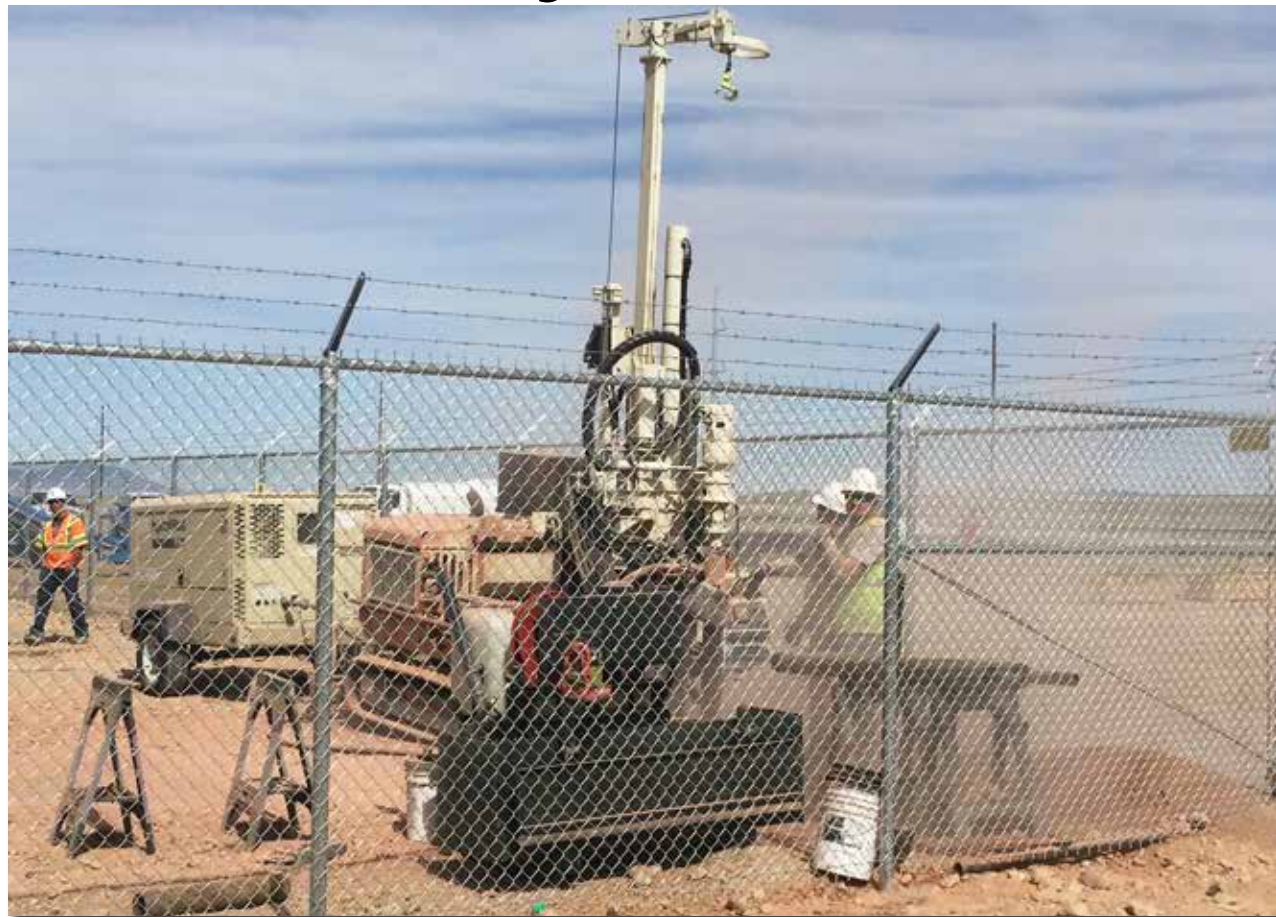
(above) The Direct Push Services field team squeezed inside the new substation area to install copper grounding rods for their project in central Utah.
