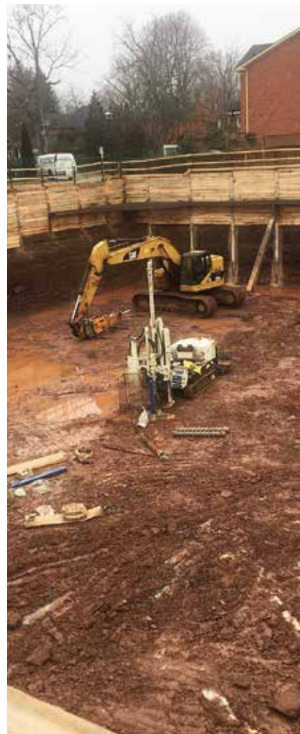
A 7822DT is lowered by crane into a shored excavation area for an environmental investigation.
