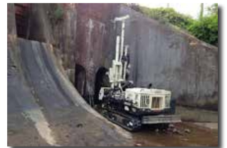
A 7822DT was lifted by a crane to complete a dam project in Aiken, SC.
