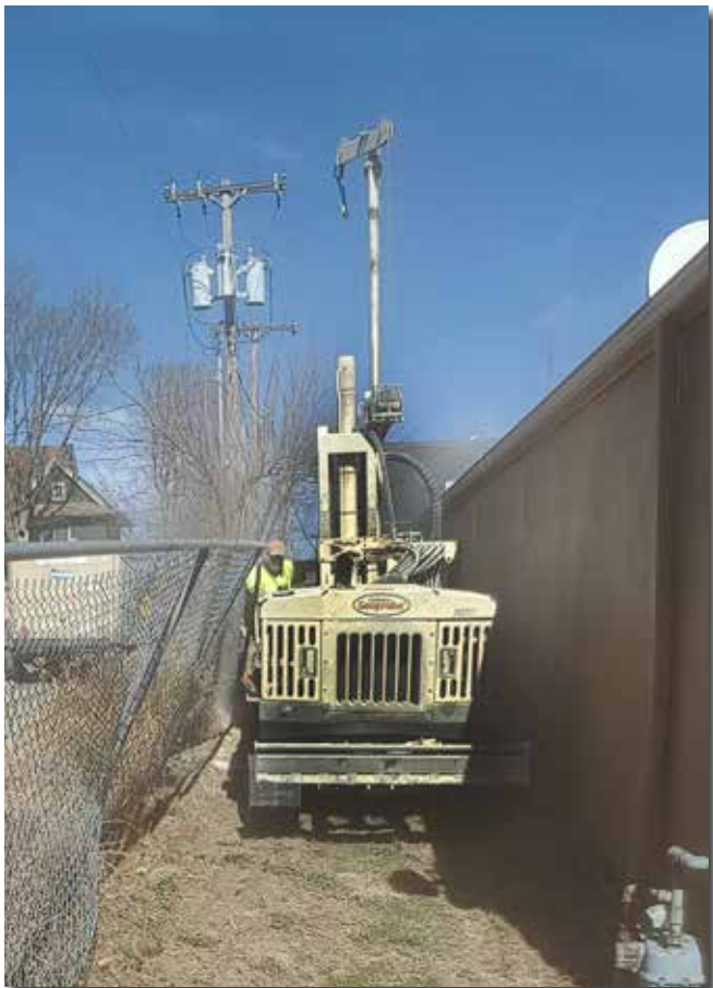
With only a 6-ft. access alley, the 7822DT had inches to spare while at some of the more confined work areas.
