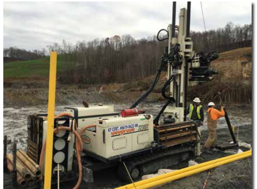
On average, the 3230DT (above) and 7822DT installed 15 to 25 dewatering points per day. Much of the variation was the result of weather and access. The contractor on site constructed "floating" roads on the ash to allow for truck and rig traffic. The roads involved placement of geo-grid material and a combination of soil and ash to a thickness of about 5- to 10-ft. to bridge over the saturated/soft ash material. This often resulted in roads that were not level.
