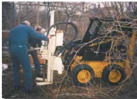
Rob Mores and his father, Rich, use the 4220 to collect soil samples on an elevated railroad embankment in Chicago. A crane lifted the machine onto the top of the embankment because of the steep side slopes.
