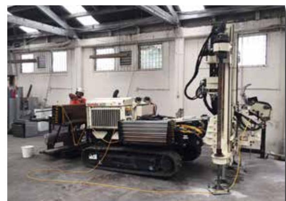
Pro-Drill fabricated a foot for the augers which they dyna-bolt to concrete slabs and foundations to perform successful pushes without cutting the concrete to screw in the anchors.
