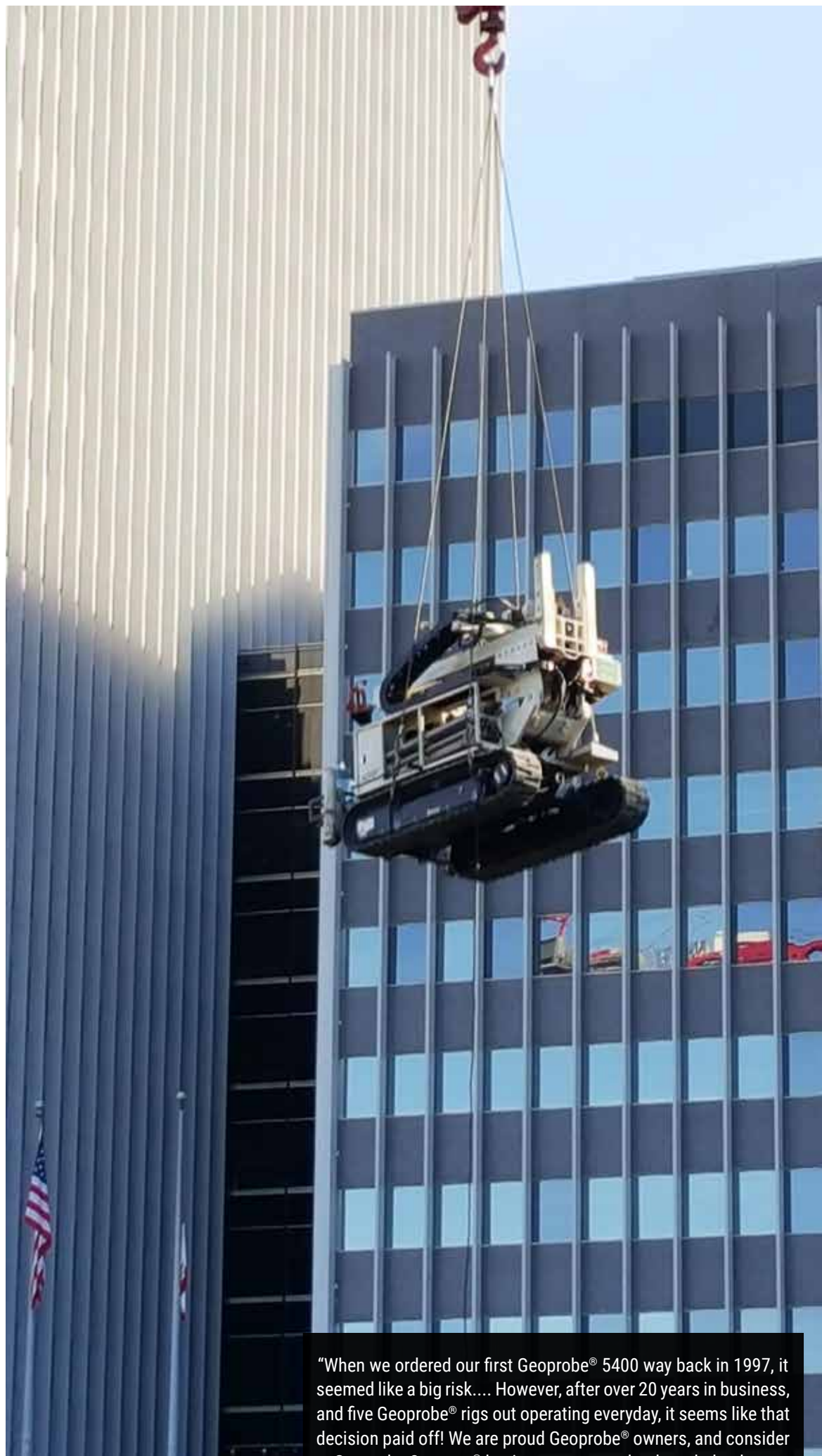
Strongarm's 6620DT flies in to help in the redevelopment of downtown Los Angeles.
