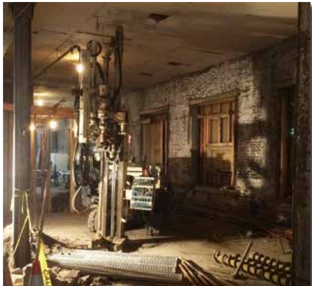
Very little head room. The vertical work space for this 7822DT, owned by Hynes & Associates in Salisbury, MD, was only 13 feet, but it was enough room to collect foundation information for structural modifications for the building.
