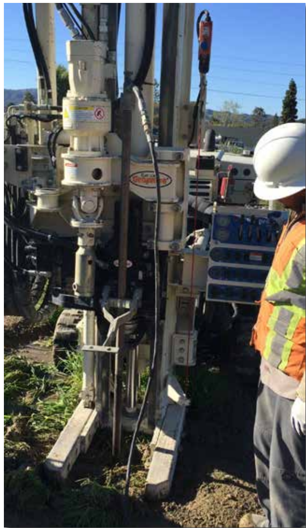
The grout mixture is pressure pumped through 1.5-in. rods using a Geoprobe® GS1000 grout machine.
