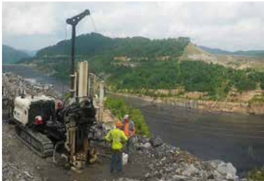
Installing PZs using PW Wireline Casing Advancers (coal refuse impoundment) with the 3230DT.
