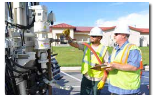
Marlan Duncan (left) and Fred Portofe, with Huss Drilling, work with a 7822DT during the injection process.
