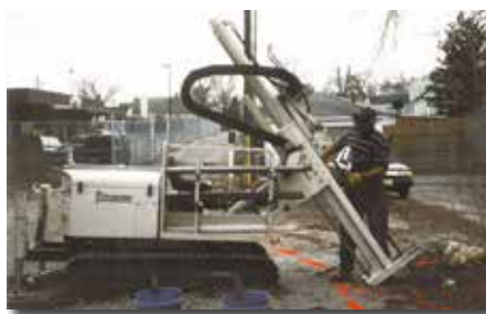
The 54DT is used to advance a series of 40 to 45 degree angled rods along a building to collect SP15 groundwater samples under the foundation.
