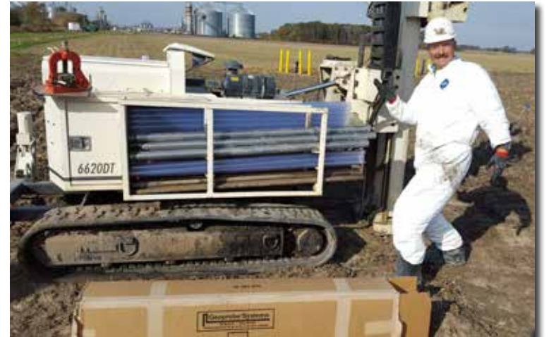
With a 100 percent retrieval success rate you'd be dancin', too! Robert Hansen, GeoServ Driller, is clearly pleased with the recovery results of the DT22 sampling system using a 6620DT.
