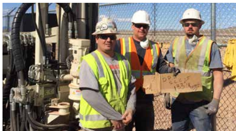
(l to r) Ryan Roodbol, Sean Bromley, and Jon Thompson drilled to 133 feet and 183 feet at all three locations to install the grounding rods.
