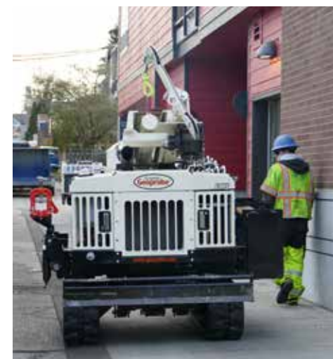
Working in the city provides a different set of restrictions for drill rigs. The compact footprint of the 7822DT helps it maneuver within the confines of alleyways and between buildings.
