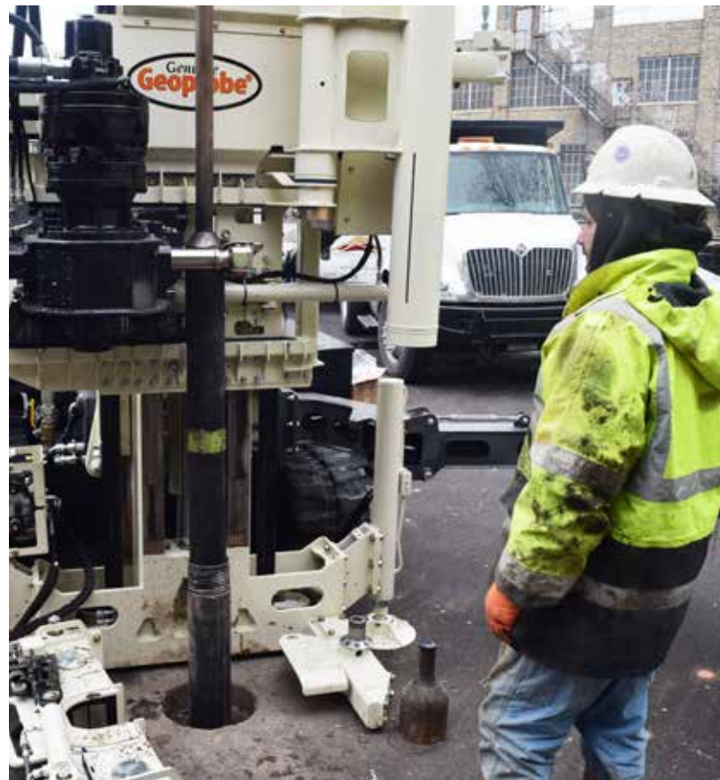
Robert Albinger uses a 3230DT to install monitoring wells in a newly paved parking lot. DT60 system was used for soil core collection and the outer casing is used for installing the well.
