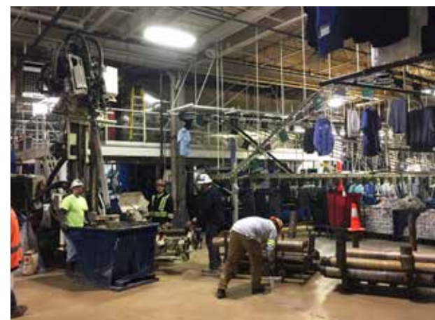
The field team was in 'full containment' mode while setting 14 bioremediation wells.
