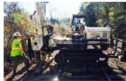
Right-of-way work on tracks near Darlington, SC. Kyle King is at the controls of Elite's 7822DT.
