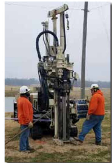
Mark Montalvo (left) and Tobin Mielenz use the Enviro-Dynamics 7822DT to perform dual tube sampling to installing 1-in. temporary wells.
