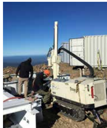
Scott Bombard, Driller, uses air rotary with a 54LT to facilitate grounding rod installation.
