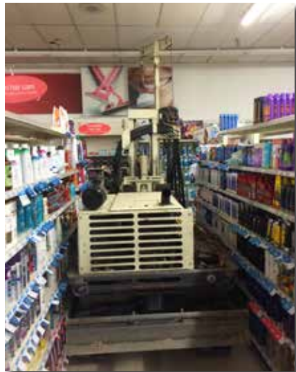
Enviro-Dynamics in Hebron, IN, uses a 6712DT with low clearance option inside a grocery store with inches to spare.
