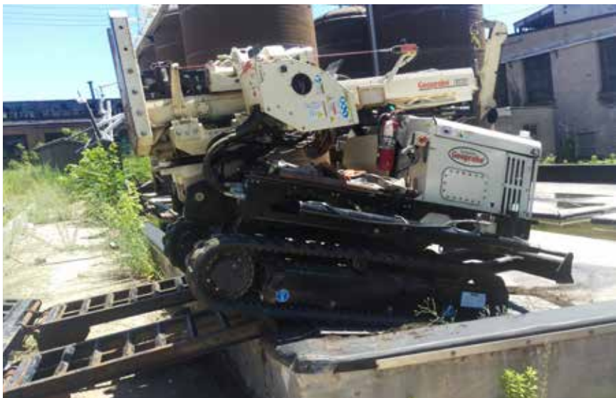
A 7822DT uses trailer ramps and soil to enter a tank farm berm at an abandoned factory in Niles, MI. Stearns Drilling was onsite to collect soil and groundwater samples.
