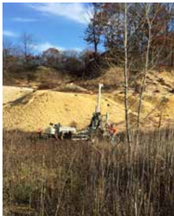
EPhase 2 uses the auto drop hammer on the 6712DT to complete geotechnical borings close to nowhere!
