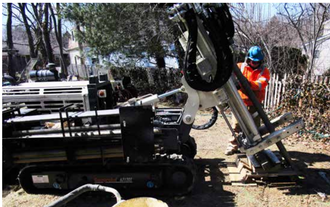
Steve Bitetto, at the controls of the 6712DT for EPhase2, installs geothermal heating and cooling systems, including direct exchange earth loops to various depths.
