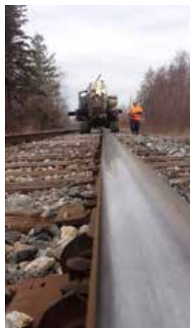
All Landshark employees are E-Rail certified for work on all Canadian Railroad lines.
