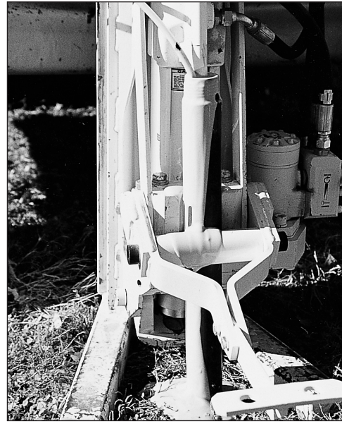
Figure 4.22. A grout machine and flexible tubing allow bottom-up grouting as the outer casing is retrieved.
