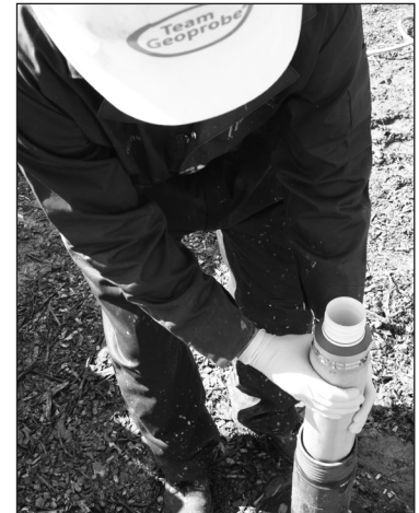
Figure 4.23. Geoprobe® prepacked screens may be installed through the outer casing when an expendable cutting shoe is used.
