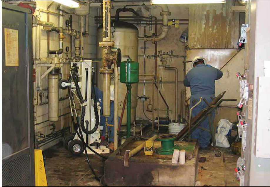
Cramped probing conditions inside building.
