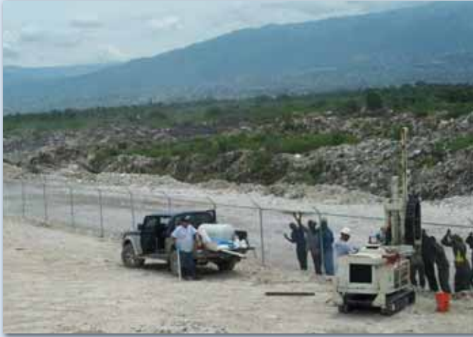
Curious onlookers. The Geoprobe® 6610DT drew a crowd while groundwater wells were installed to assess the water quality at the Truitier Landfill. Ernesto Garcia (white hard hat), Drilling Assistant for Enviro Tek, operates the rig.
