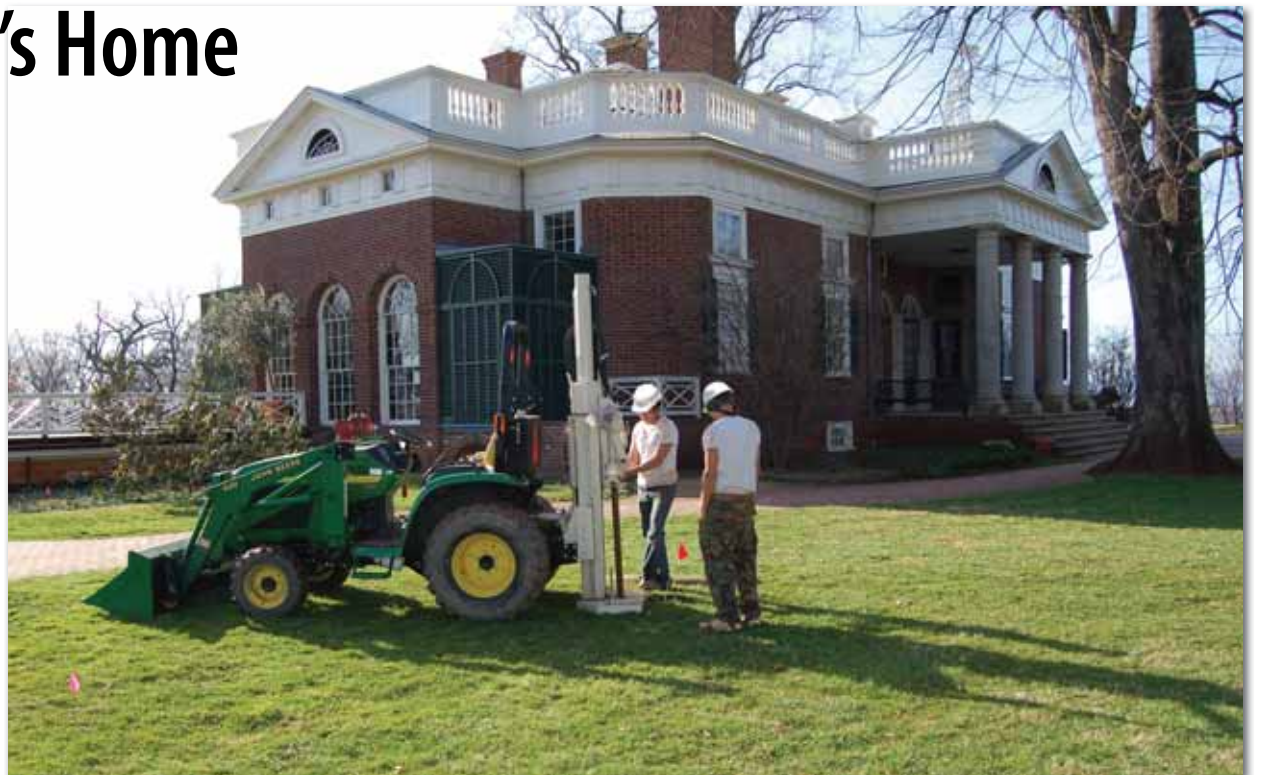
Indiana University students Joel Marshall (left) and Luke Walker use the 54TR on the East Lawn at Monticello to collect discrete soil samples using DT22 tooling. The samples will help document 18th century landscape modifications made by Monticello's former resident, President Thomas Jefferson. It's all part of the Monticello Plantation Survey, a long-term effort to complete an inventory of the archaeological resources located on the 2,000-acre tract currently owned by the Thomas Jefferson Foundation.
