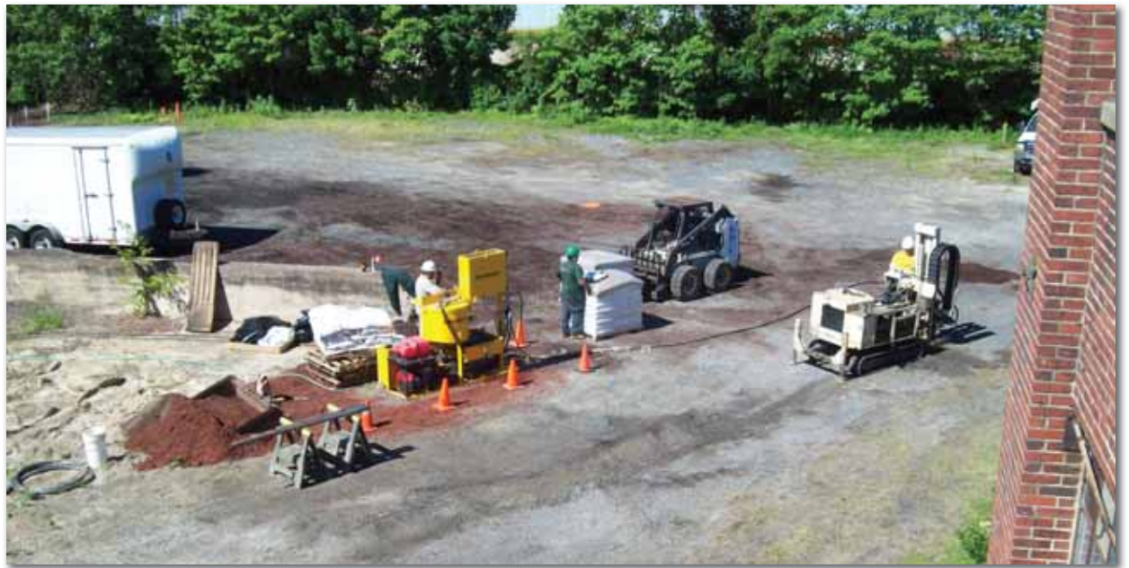
Approximately 60,000 gallons of EHC ® slurry was injected during a 30-day period at a TCE contaminated site in New Jersey. An EHC ® slurry was injected in grid patterns across three main targeted areas with approximately 400 gallons of slurry injected per location.
