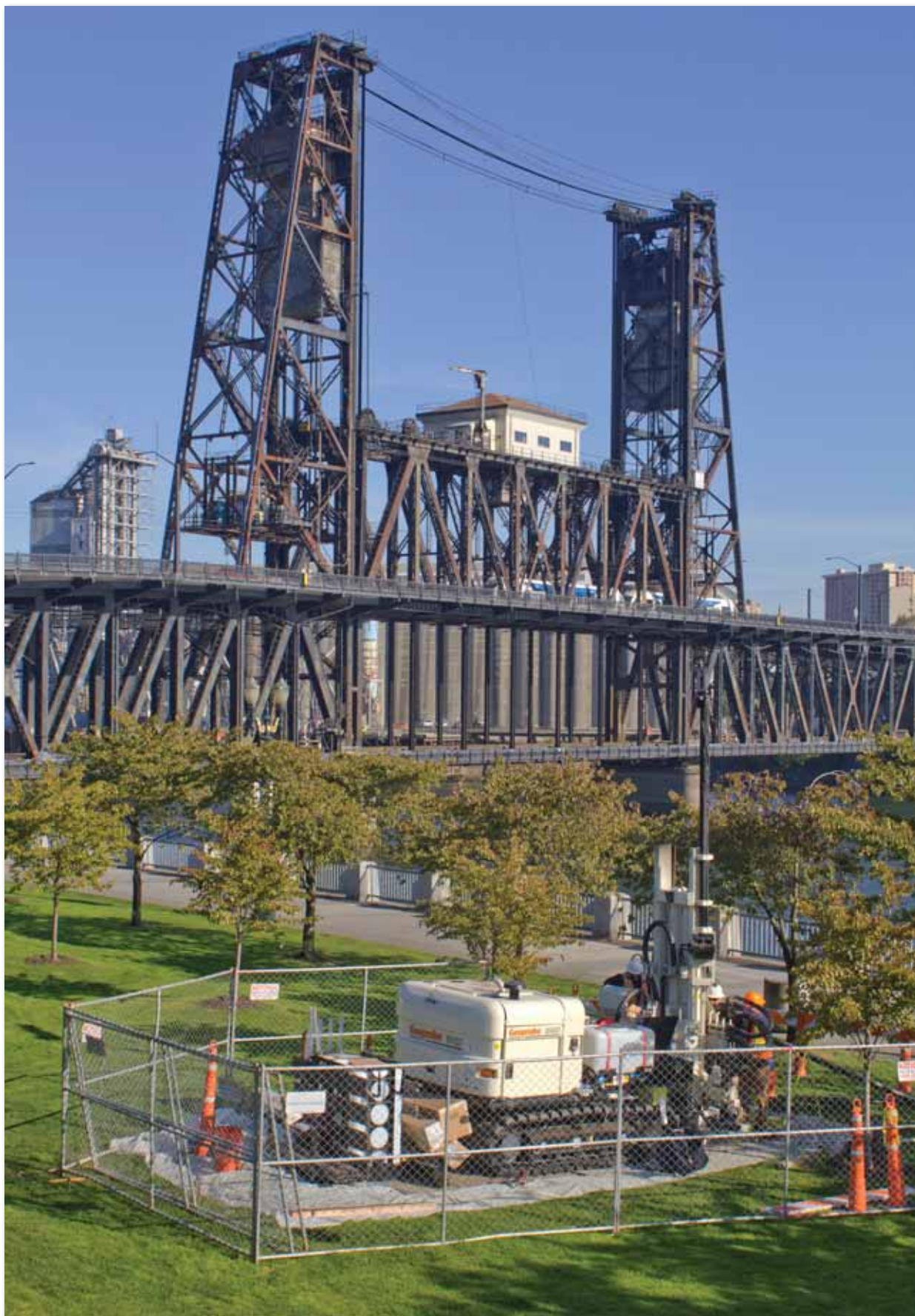
The Cascade Drilling field team used protective mats under the 8040DT to minimize site impact. The Geoprobe® Drop Rack System was also used for tools and supplies transport to minimize the number of trips made back and forth to the support vehicles. And because the park is such a popular area for Portland residents, protective fencing was installed to ensure the safety of the public. The Steel Bridge over the Willamette River can be seen in the background.
