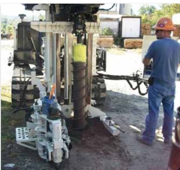
Chris Henderson, Driller for EnviroProbe, uses 6-5/8 in hollow stem augers to install an extraction well.
