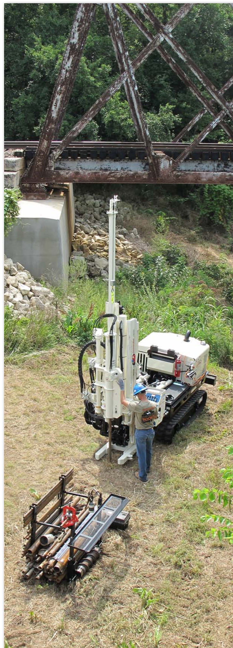
Using the automatic drop hammer on the 7822DT to gather SPT blow counts.
