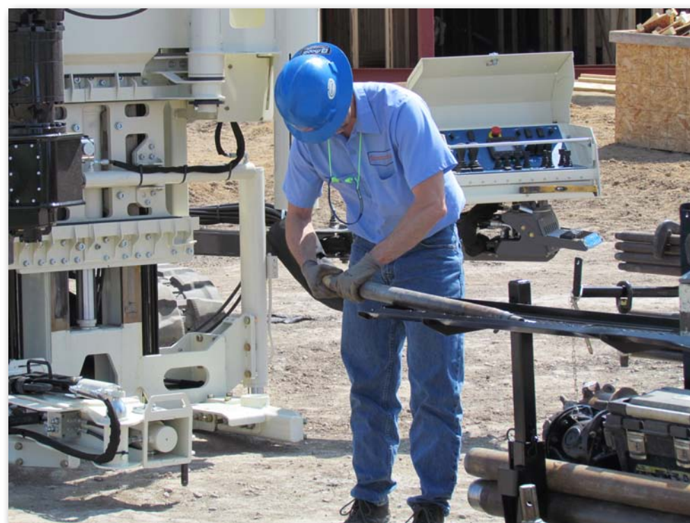
Taking SPT split spoon samples with the new 3230DT at a construction site.
