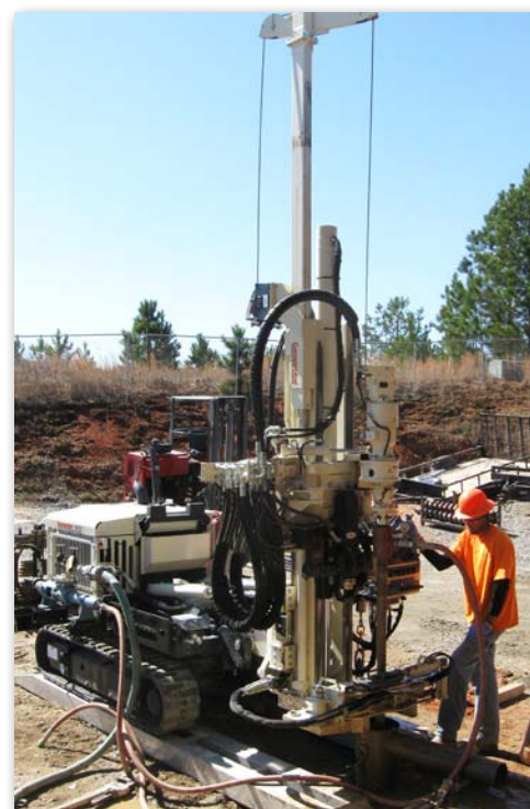
During monitoring well installation, Scudday Horner advances a tricone roller bit with a 7822DT while circulating mud with a Moyno® pump to stabilize the borehole.
