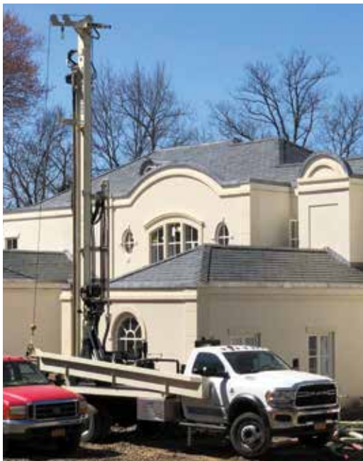
At a limited-access residential site in New York, the DM250 efficiently completes 15 bores to 305 feet through tough, plastic clay 80 percent of the hole to install geothermal field at a large residence.
