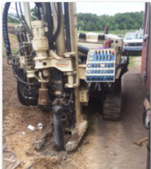
As part of the closure of a former underground storage tank at the Big Sandy Wastewater Treatment Facility, Geo Logic used a 7822DT to set a 2.0-in. monitoring well through 4.25 in. hollow stem augers.
