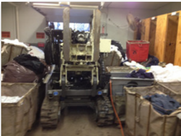
With just under 12-ft. overhead clearance, Enviro-Dynamics in Hebron, IN, will use a 6712DT to install a monitoring well to 25 feet inside a dry cleaners facility.
