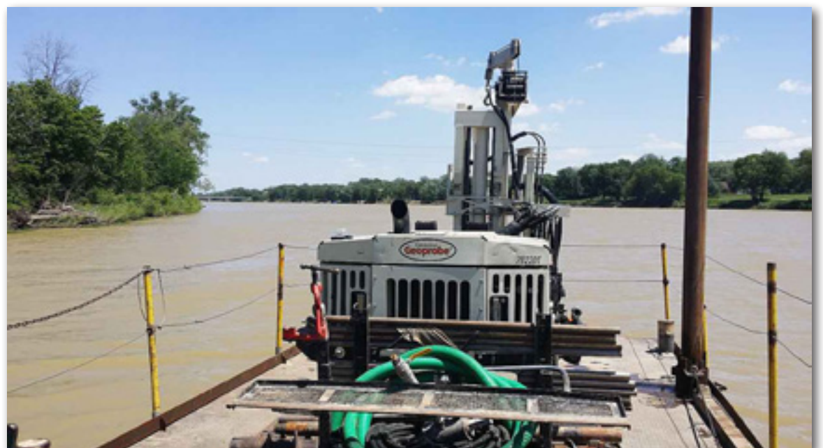
A 7822DT, owned and operated by Mannik Smith Group, heads down the Maumee River for the start of a geotechnical investigation to help determine a new river crossing for US24/US6 arterial corridors for residents and local businesses, including the world’s largest Campbell’s Soup plant. The new bridge will provide a vital direct link between two industrial/office park areas of Napoleon/Henry County in Ohio.
