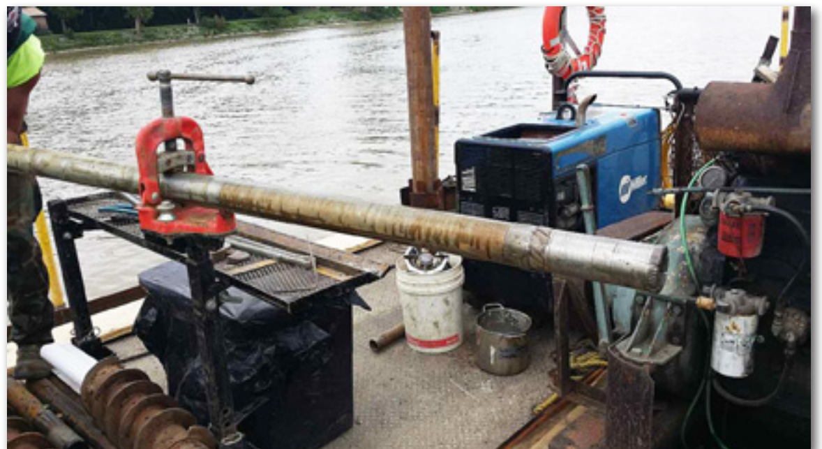
MSG used a 7822DT to complete 26 soil borings totaling 353 linear feet, including a total of 150 linear feet of rock coring using an N-sized core barrel. The type of rock cored was mainly dark brown to black shale, slightly-to-moderately-weathered, thinly laminated, weak to moderately strong.
