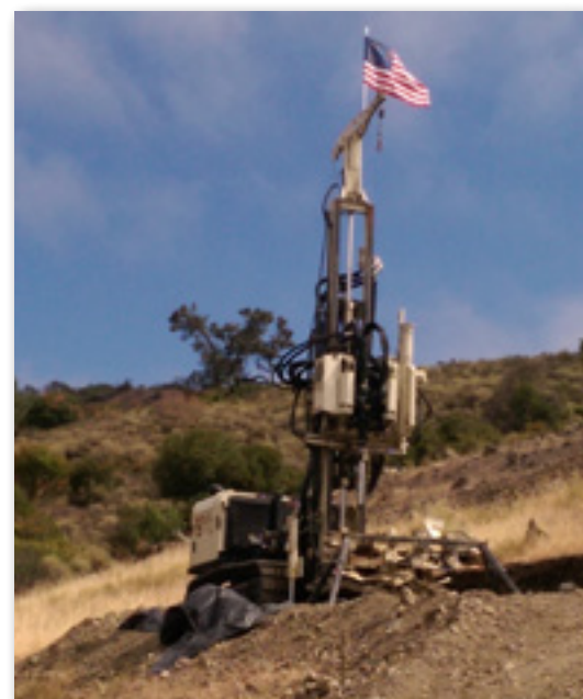
The 8140LS Sonic at a California dam site near San Jose.
