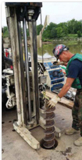
Rob Schippert, MSG Lead Driller, advancing 4.25 in. hollow stem augers for a riverbed boring.
