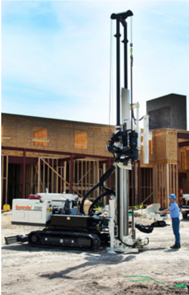
The telescoping mast, with a maximum height of 23 ft. 10 in., allows the field team to trip 20-ft. sections of tooling.
