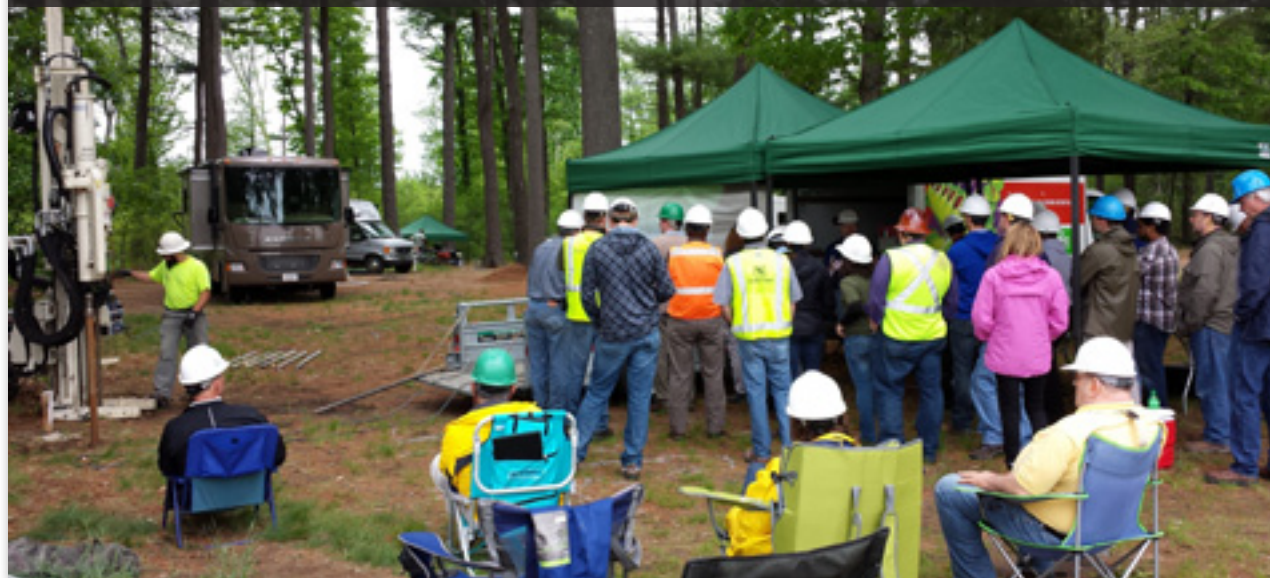
Al Allen, with Crawford Drilling Services in Gardner, MA, advances an MiHpt probe using a Geoprobe® 7822DT during a field demonstration for the Massachusetts Licensed Site Professional Association (LSPA) outside of Boston, MA. Under the tent, Dan Pipp, Geoprobe® MIP Specialist, describes details of the LL-MiHpt Logging System and its operation to the seminar attendees.
