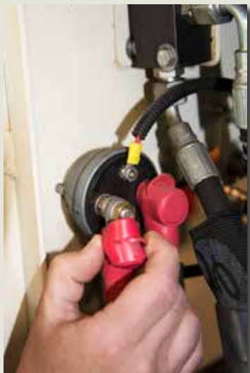
Master Disconnect on 8040DT.
