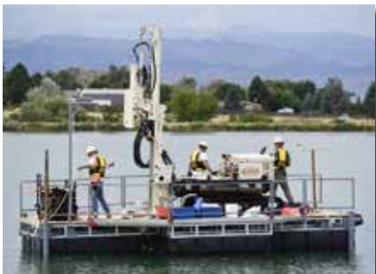
Drilling Engineers designed a barge to accommodate their Geoprobe® 7822DT for the geotechnical investigation on Erie Lake Reservoir.
