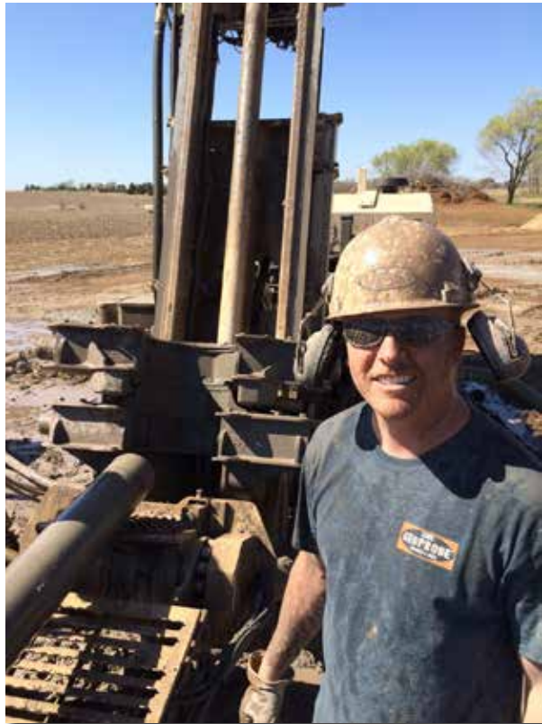
Jed Davis, Geoprobe® Tooling Engineer, takes testing rigs and tooling seriously ... it's not for the faint of heart! Jed is running 6-in. casing using the 14-in. breakout with 9-in. vertical travel. The breakout has an adjustable clamp force of 0 to 21,000 lbf and 14,500 ft-lb of torque.
