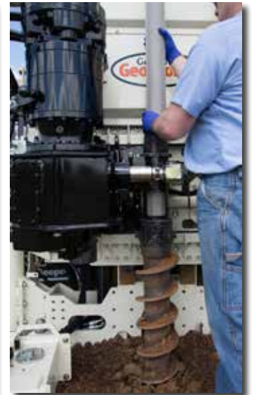
Pulling 4.25-in. hollow stem augers with open ID to simplify well installations.
