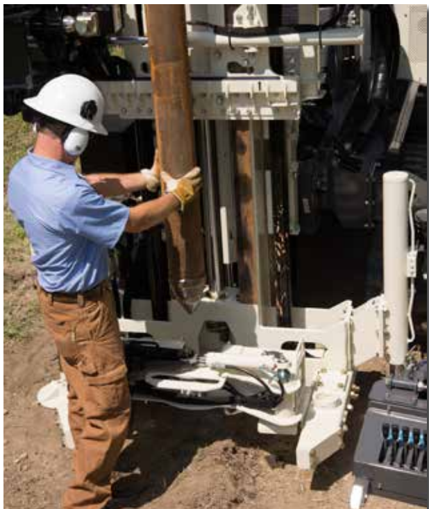
These machines do NOT lack power! Drive 6-in. casing. Get your augers down. This machine is going to produce for you.
