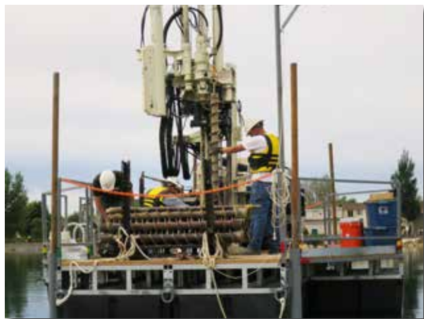
Drillers for Drilling Engineers use 3.25 in. hollow stem augers with their 7822DT machine on a barge on Erie Lake Reservoir.
