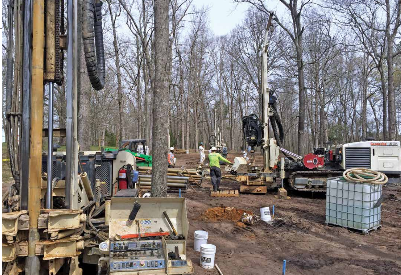
SAEDACCO uses 8140LS and 8150LS to pre-drill borings using 4X6 system 122 feet to 170 feet below ground, conducting continuous logging in 10 percent (top). AST Environmental uses their 7822DT to inject 60,000 lbs of BOS 100® through 2.25-inch rods (bottom).
