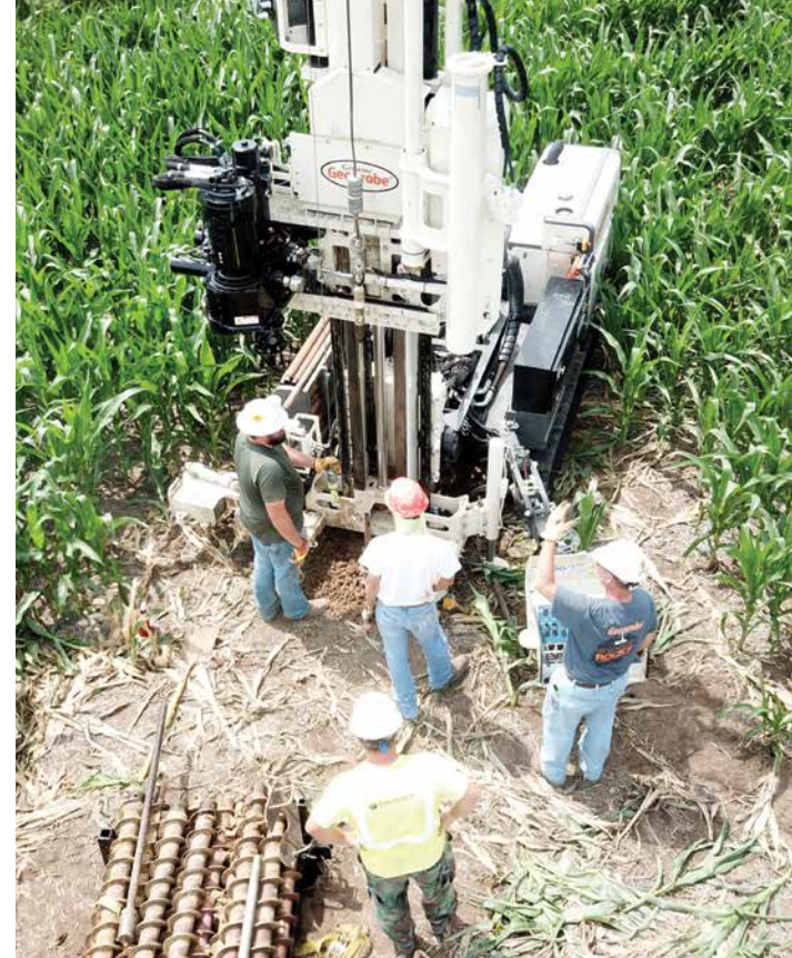
Flooding has kept the Nebraska Department of Transportation busy completing bridge foundation and slope failure tests, increasingly relying on CPT to inform designs (top left). With the versatility of the 3230DT they create less mess, exert less energy, and complete projects faster (above).
