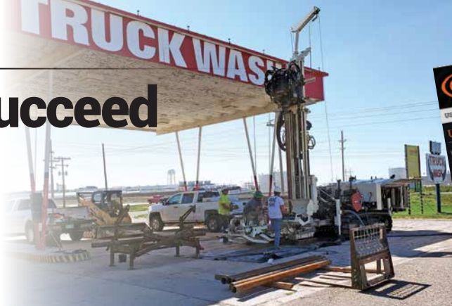
Geoprobe® 8150LS sonic successfully dry drills to 200 feet in tough formations in Oklahoma.
