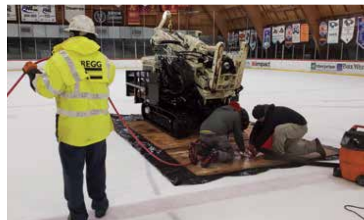
The spacing between the piping was very close to the tooling, so drive caps were wedged in between to spread the piping apart (left). The ice was melted by the rink staff with the use of warm water and a wet-dry vacuum to expose the polyethylene refrigerant piping. Gregg Drilling LLC had to keep the water hose elevated or moving to prevent melting grooves in the ice (below).
