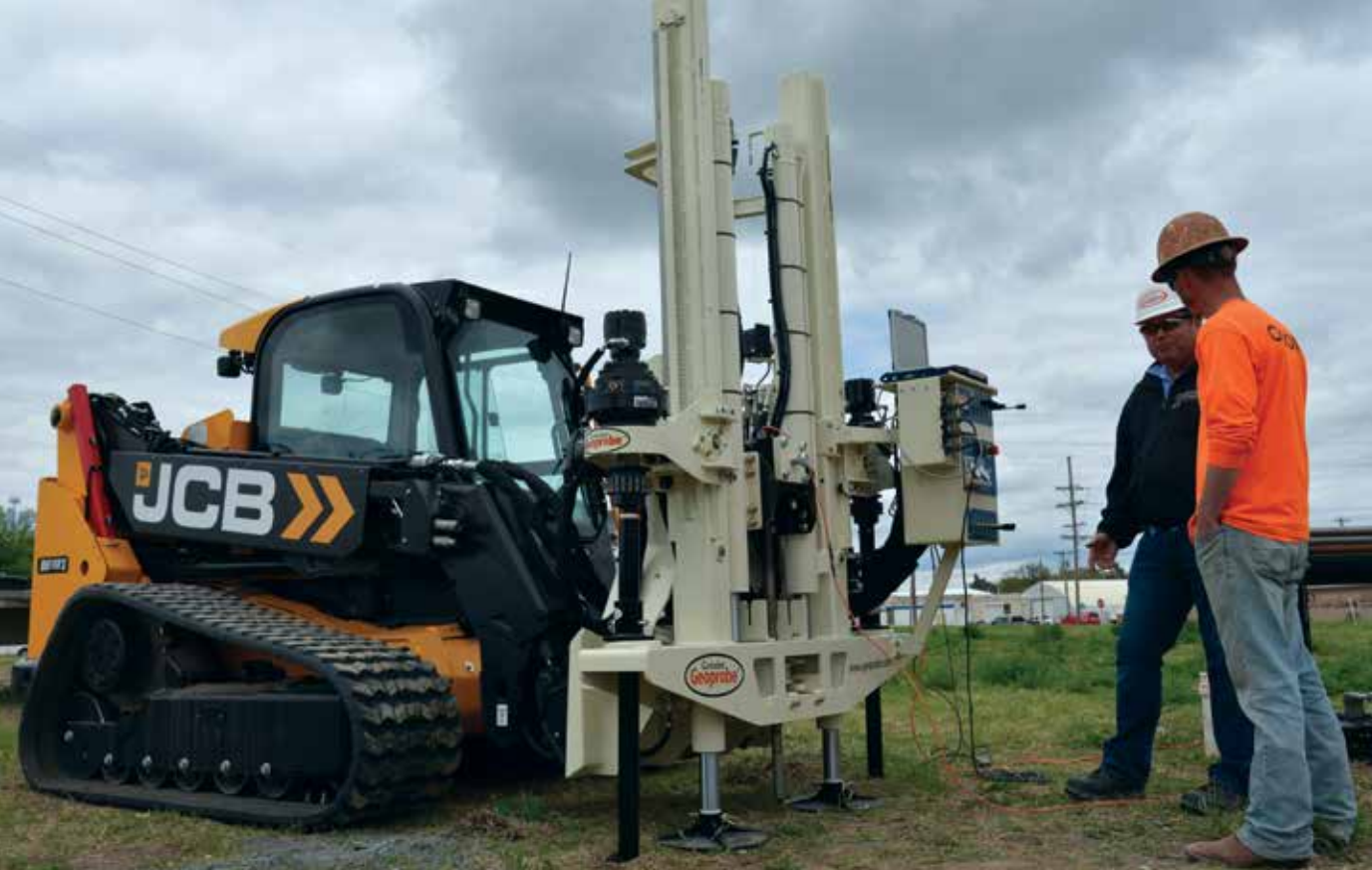
Whether it's in the field or at Geoprobe® headquarters in Salina, training is key to getting the most out of your CPT efforts with Geoprobe® machines. In order to maximize return on their CPT investment and ultimately meet customer needs, Kevin Whitla (right) of Olsson Inc. in Lincoln, Nebraska, trains with Troy Schmidt (left), following the purchase of their new Geoprobe® 20CPT Press.
