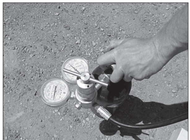
Fig. 7.10. Nitrogen gas cylinder main valve.
