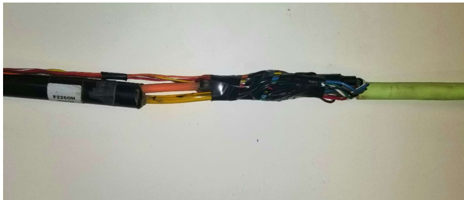
Figure 4.7 Looped OIP Trunkline Leads
