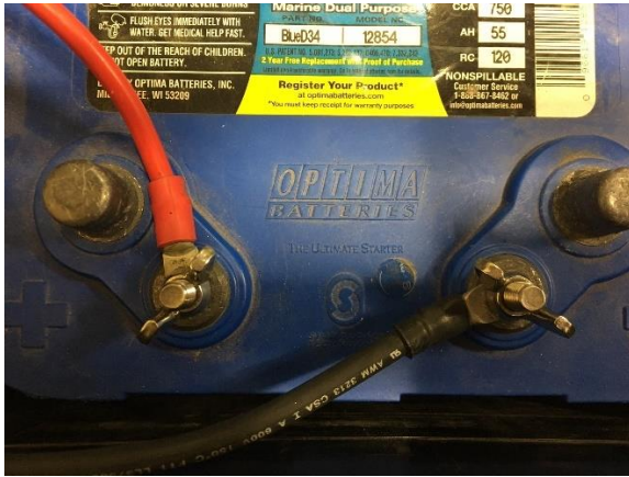
Figure 15: Connection Between External Battery Cable and External Battery.
