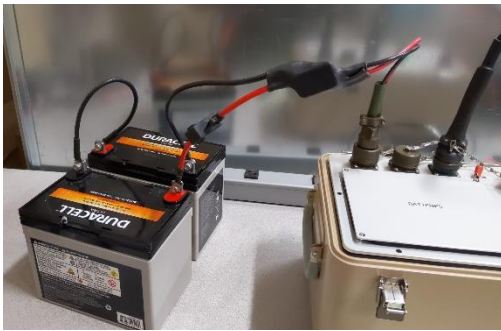
Figure 13: Connection of external 12V batteries in 24V supply configuration.
